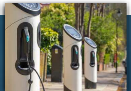
EV Charging Points
